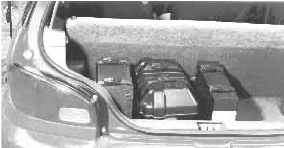
Figure 18 — The 500-watt system fits neatly in the rear compartment of the GEO Metro
